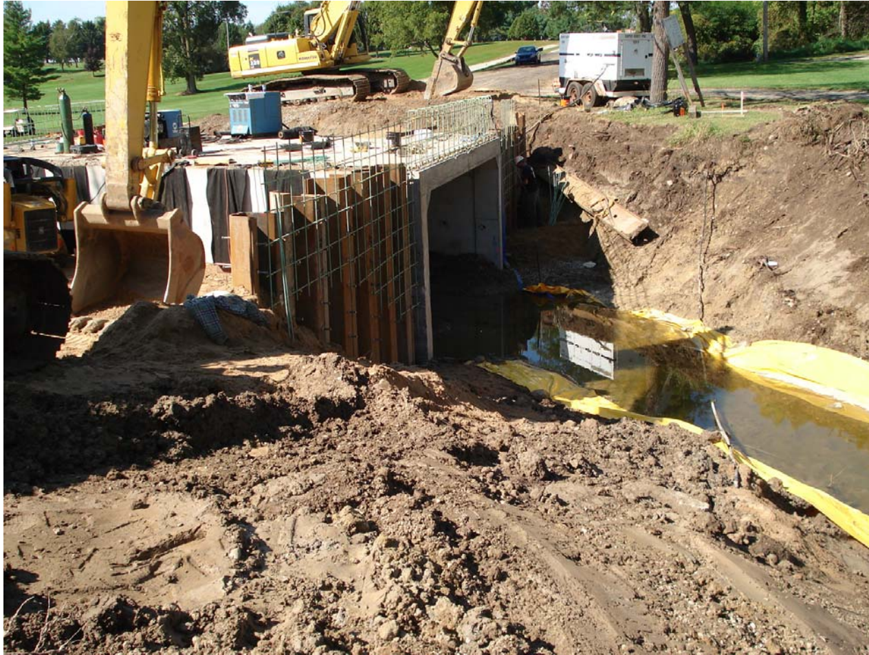
North end of culvert – No slope protection/silt fencing Turbidity Curtin being used as slope protection
